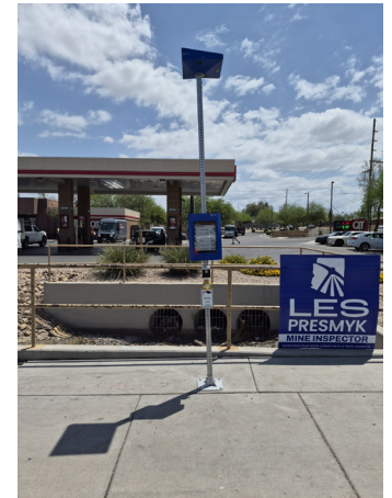
Pole Mounted Lightining during day .
